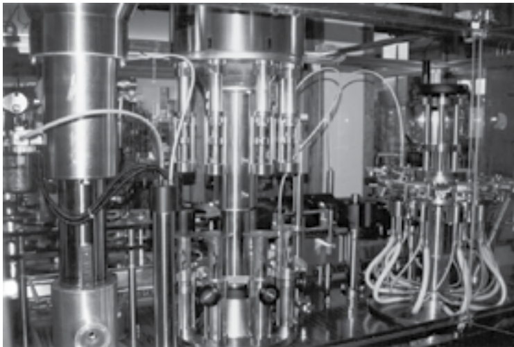
Equipment in a commercial food-processing facility is generally made of stainless steel, which allows for adequate cleaning and sanitizing.
